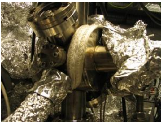
Figure 5.3 View of the Bakeout setup.
